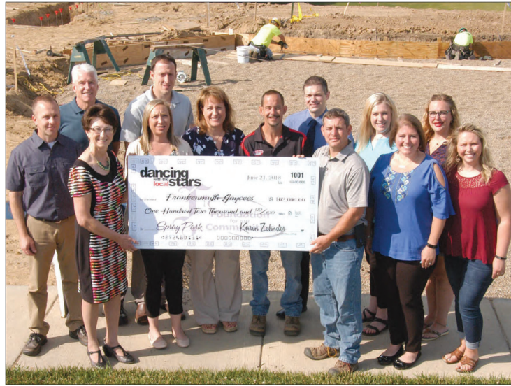
DANCING DOLLARS! The Dancing with the Local Stars committee gathered at the site of the under-construction Frankenmuth Spray Park, located in Memorial Park. The nearly $1 million project is spearheaded by the Frankenmuth Jaycees, with fundraising coming from various community organizations and residents. The committee met on Thursday, June 21, to officially award the Jaycees with a check for $102,000. The funds were raised in the last four years of Dancing with the Local Stars, held at the Bavarian Inn Lodge. The committee would like to thank everyone who has helped to make this fundraiser happen since it began in 2015. "This event would not have been possible without the dedication and effort put in by our dancers, judges, DJ, master of ceremonies, donors, attendees and our committee these past years," Dancing with the Local Stars Committee Chair Karen Zeindler said. There will be one more Dancing with the Local Stars event, set for Saturday, March 9, 2019, at the Lodge. All proceeds will continue to be earmarked to improve recreation in Frankenmuth. (News photo)
